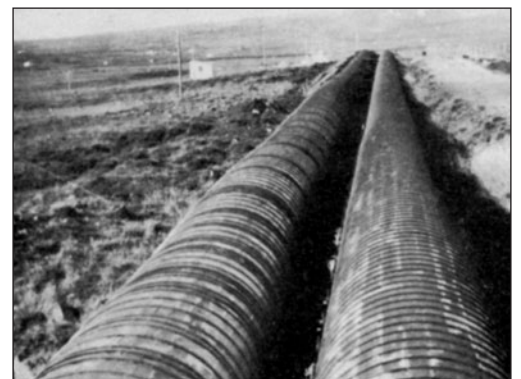
Wooden pressure pipes leading water into the turbines. Lake Ellidavatn was the reservoir.
