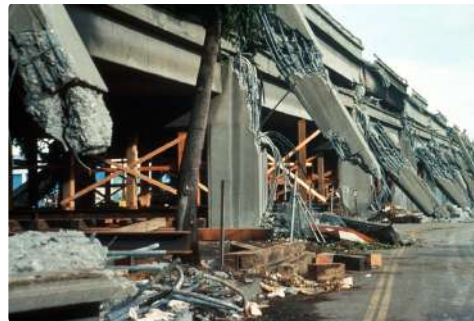
A highway on two levels, that collapsed in the Northern California earthquake of 1989
